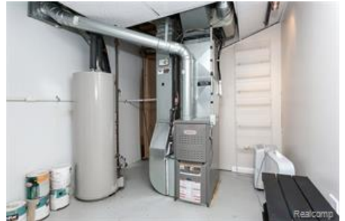
Updated Furnace and Water Heater Maintained by Co-Op
