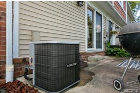
Brand New Air Conditioner (2019)
